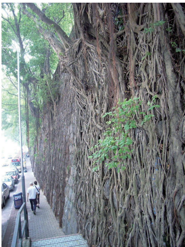
图2 地表根覆盖于挡土墙形成“树墙” Fig.2 The ground roots cover the retaining wall to form a ‘Tree Wall’
